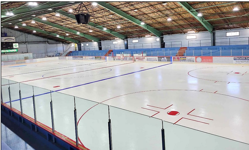
The ice surface after a temporary dehumidifier was installed, repairs to the ice and line painting were completed.
