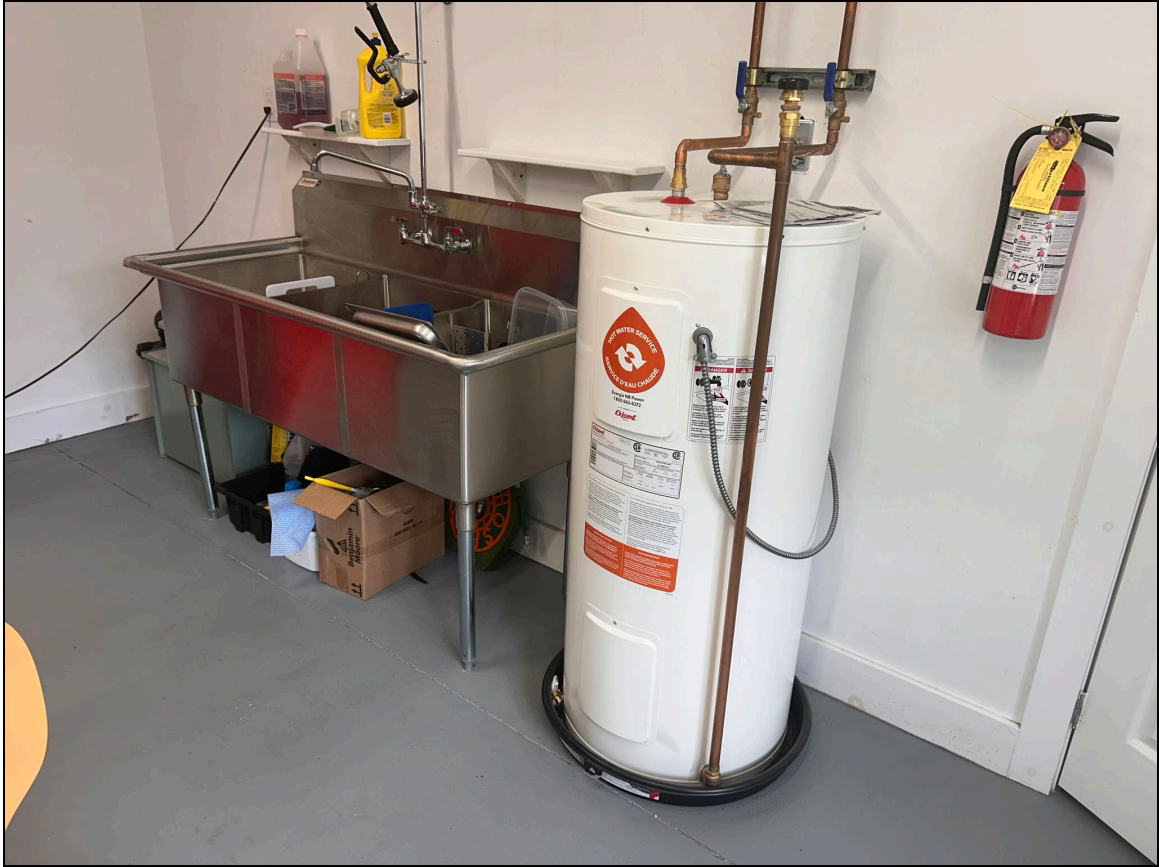
Interior, 3 sink wash area and hot water heater.
