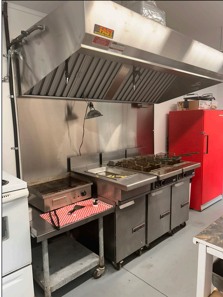
Interior, municipal owned deep friers and exhaust system. Other items such as appliances are not included in this agreement and are responsible for the proponent/operator.
